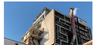
Chemical recovery boiler
